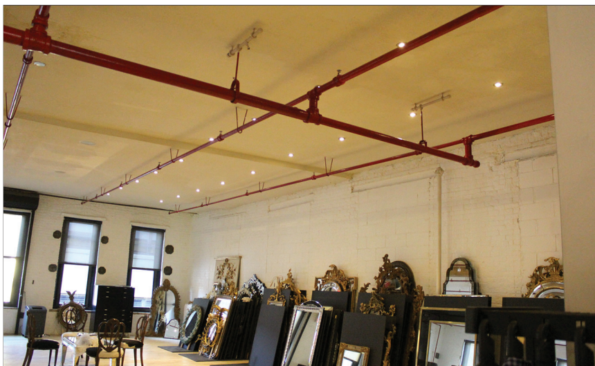
Figure 5-20. Fire protection piping and sprinkler heads installed along the building ceiling.
